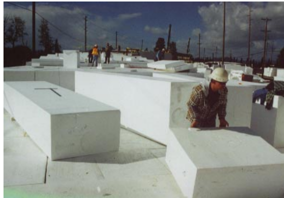
An Ostrander Rock & Construction worker moves Geofoam blocks into place. Each 16 foot-long block weighs approximately 280 pounds.
