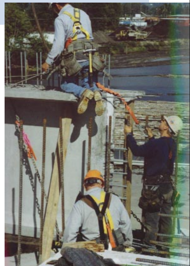
Five Rivers Construction workers steady the first of seven pre-cast concrete girders as they are moved into place atop the Fibre Way Grade Separation project.
