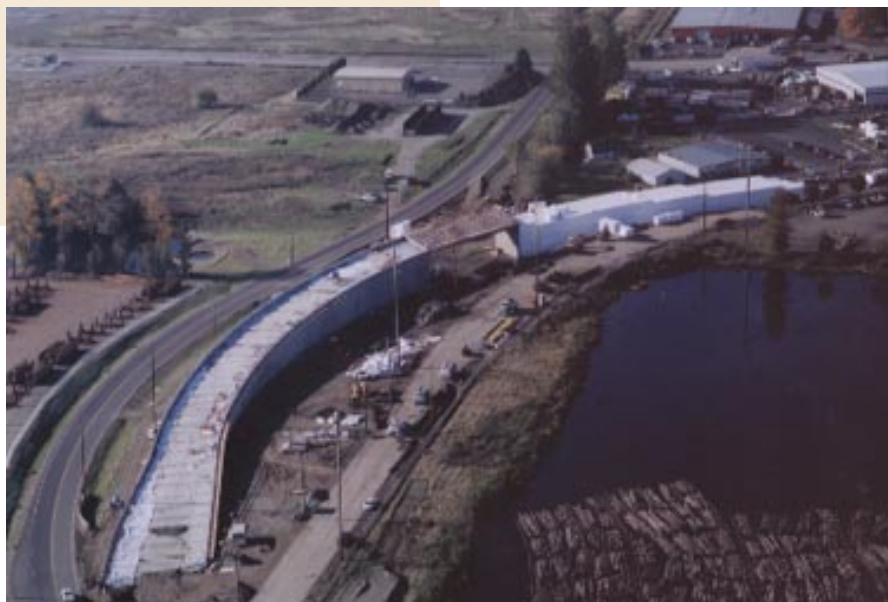
Fibre Way Grade Separation project under construction in November 2001. Geofoam fill can be seen at the top right.
